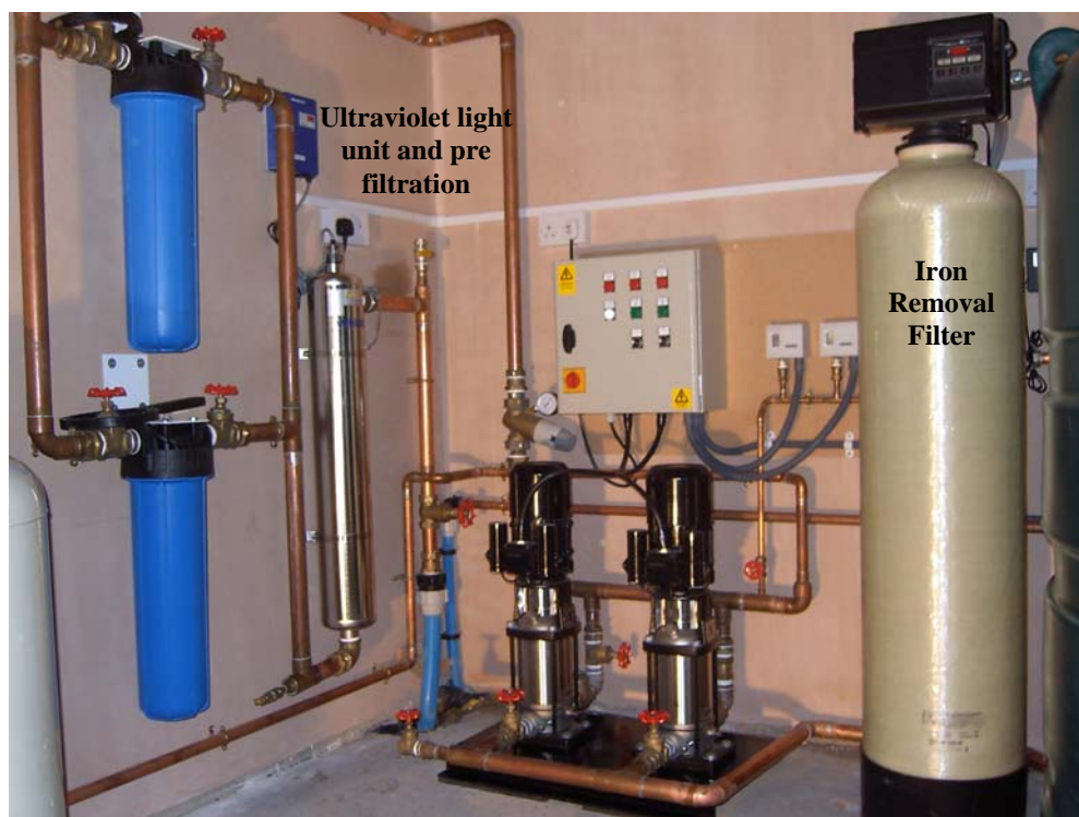
Typical Iron removal filter installed in a plant room serving a large residential property
